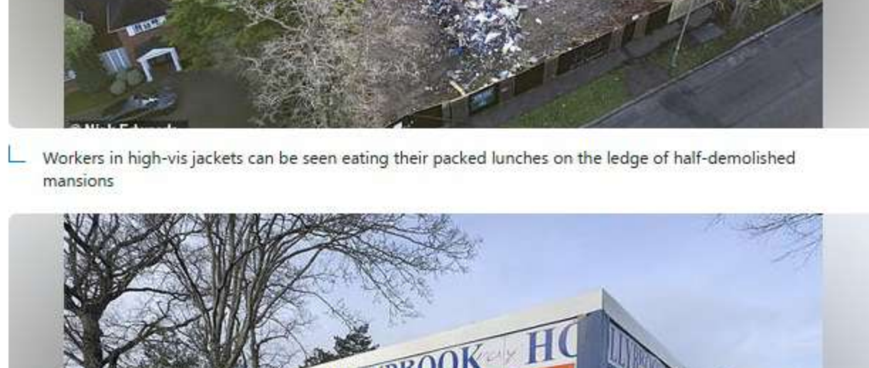
Workers in high-vis jackets can be seen eating their packed lunches on the ledge of half-demolished mansions
